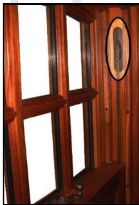
Fig 1: Window Pulley Circled Above
